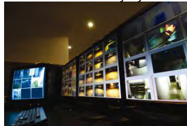
Industrial Security Systems
